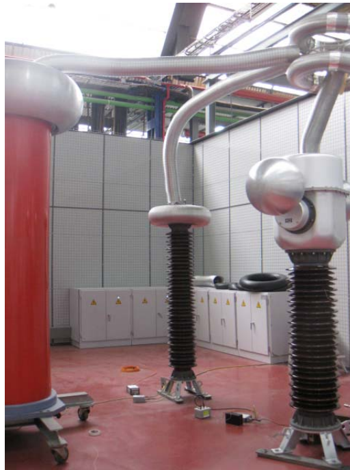
Routine tests in ARTECHE's installations.
